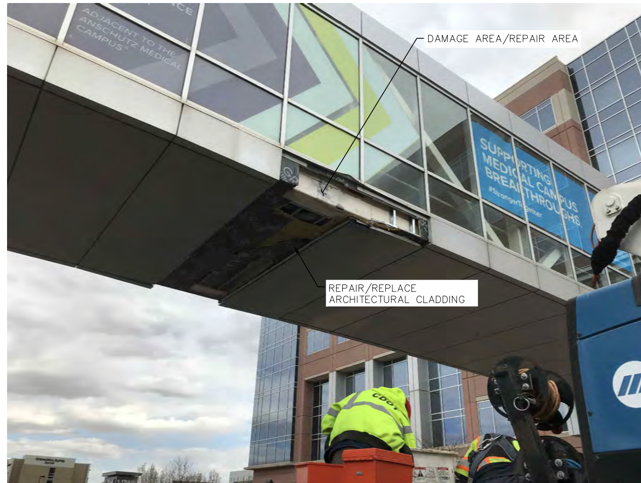
LOCATION OF DAMAGE IN WESTBOUND LANES E COLFAX AVE LOOKING SOUTHEAST
